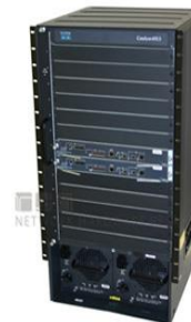
Ethernet switch (Cisco Catalyst 6513)
